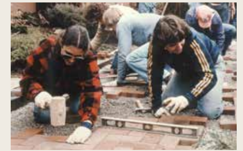
1985: Students in the nursery management major retrofit brick pavers into the Earth Science Center patio garden, installed by the first graduating class in 1973.
